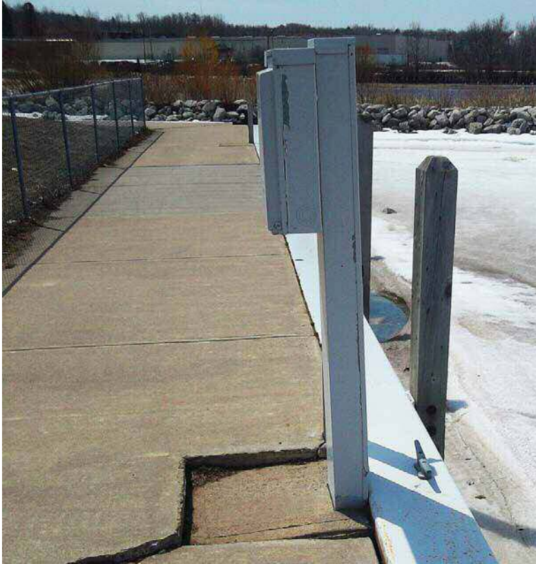
Photo 17: Typ. Power Pedestal
