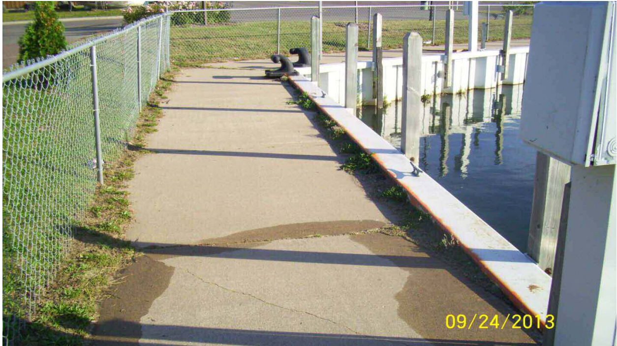
Photo 21: Settled sidewalk at NE corner
