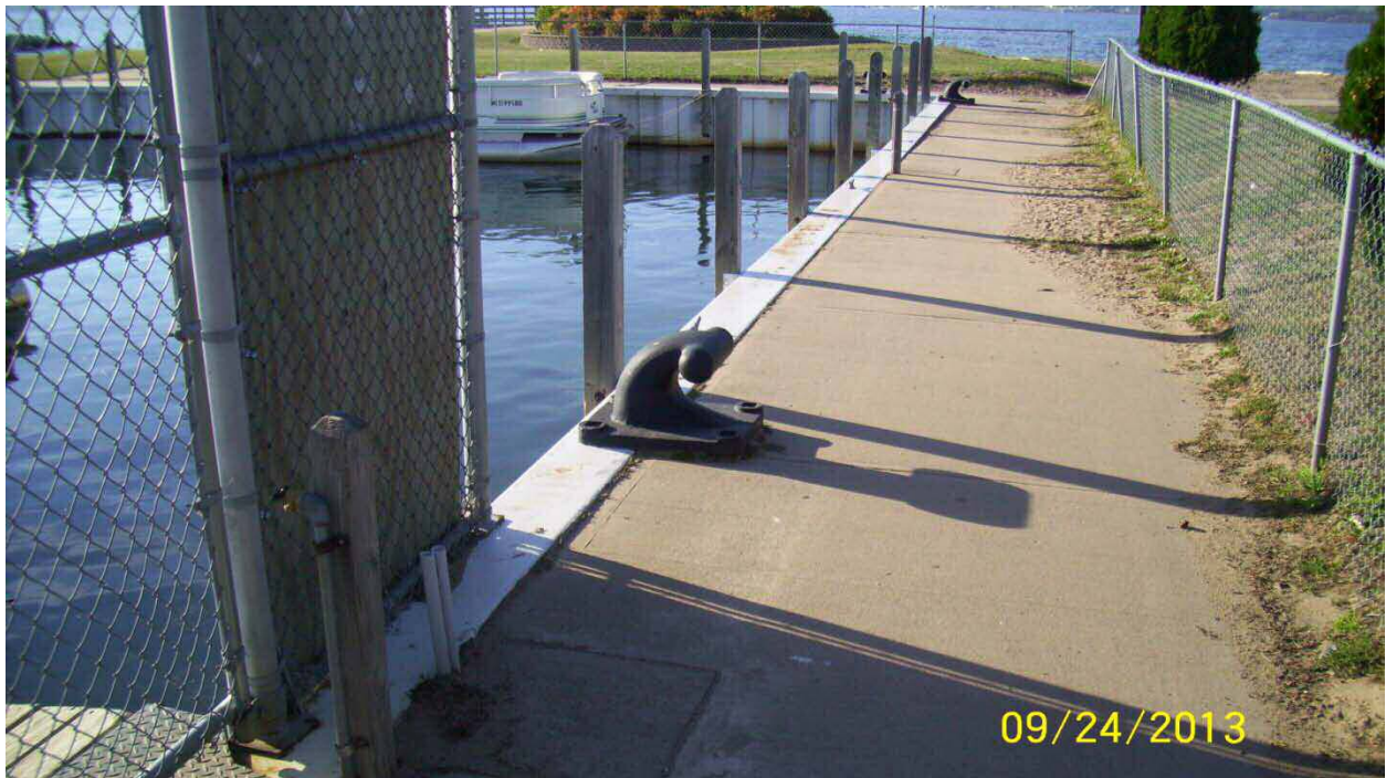
Photo 20: Sidewalk at north has settled near fence
