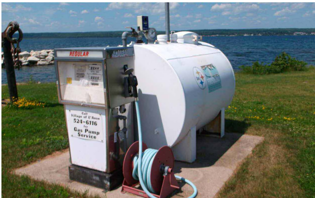
Photo 14: 500 gallon fuel tank & pump (not active)
