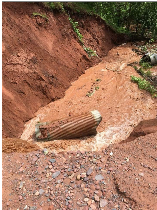
Trail washout after the Jun 17, 2018 Houghton flood. Photo courtesy of Keweenaw ATV Club.
