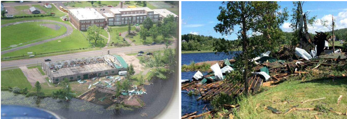
Straight line wind damage on July 11, 2016 tore the roof off the old skating rink in Wakefield and destroyed outbuildings (Photo: NWS Marquette and Michigan State Police).
