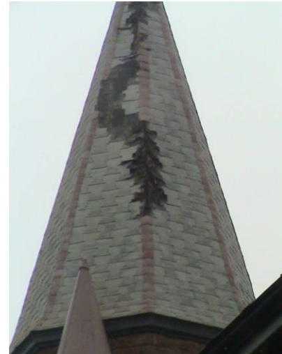
2013 lightning damage to St. Anne's Church in Calumet (Photo: Keweenaw Heritage Center)
