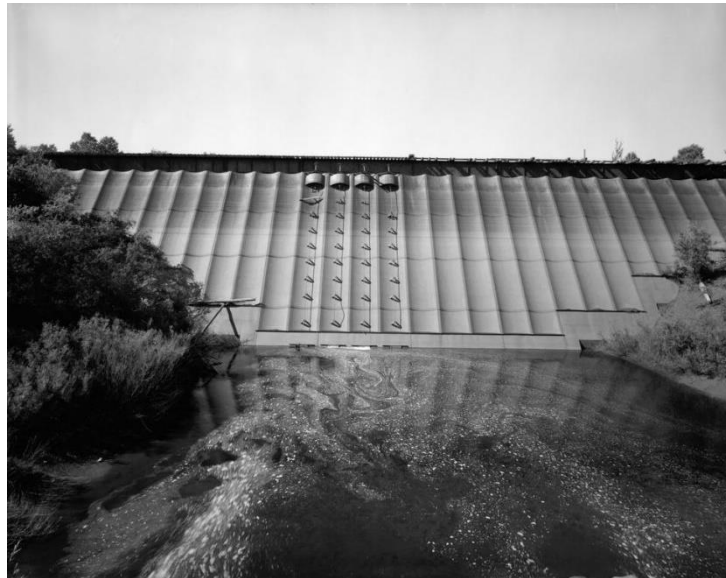
The image above was found at the Library of Congress HAER archive entry with the original caption: "VIEW LOOKING AT UPSTREAM SIDE OF DAM. HAER MICH,31-BEHIL,1-1" It is a part of the Historic American Engineering Record collection of photos. Redridge Steel Dam, Houghton County, Mi, image taken by Jet Lowe, HAER photographer, in July 1978.
