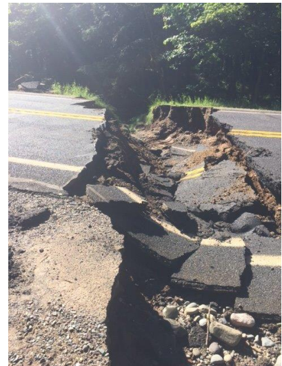
M-73 culvert washout on June 11, 2017 (Source: MDOT (NWS Marquette) )
