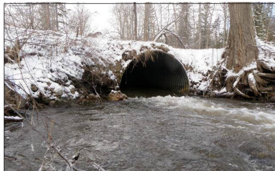
Upgraded culverts can mitigate flooding problems by increasing the flow capacity of streams as they pass under roadways.
